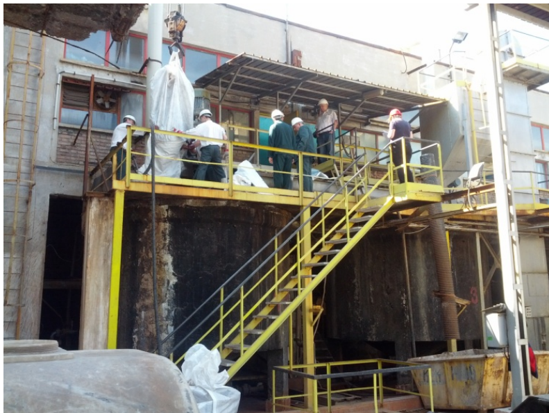
Figure 3. Industrial testing facility, KCM 2000, Plovdiv, Bulgaria
