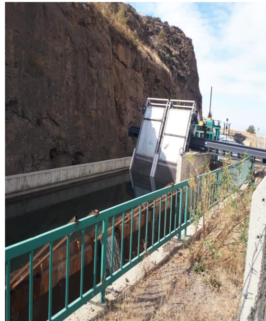
Figure 6b. Mechanical bar screen field application
