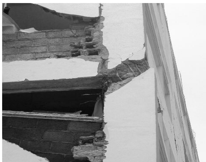
Figure 3. Shear collapse due to the interaction between masonry and frame in Boumerdes town.
