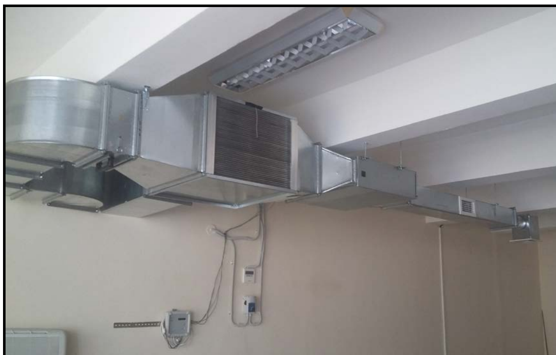
Figure 2. General appearance of air handling unit
